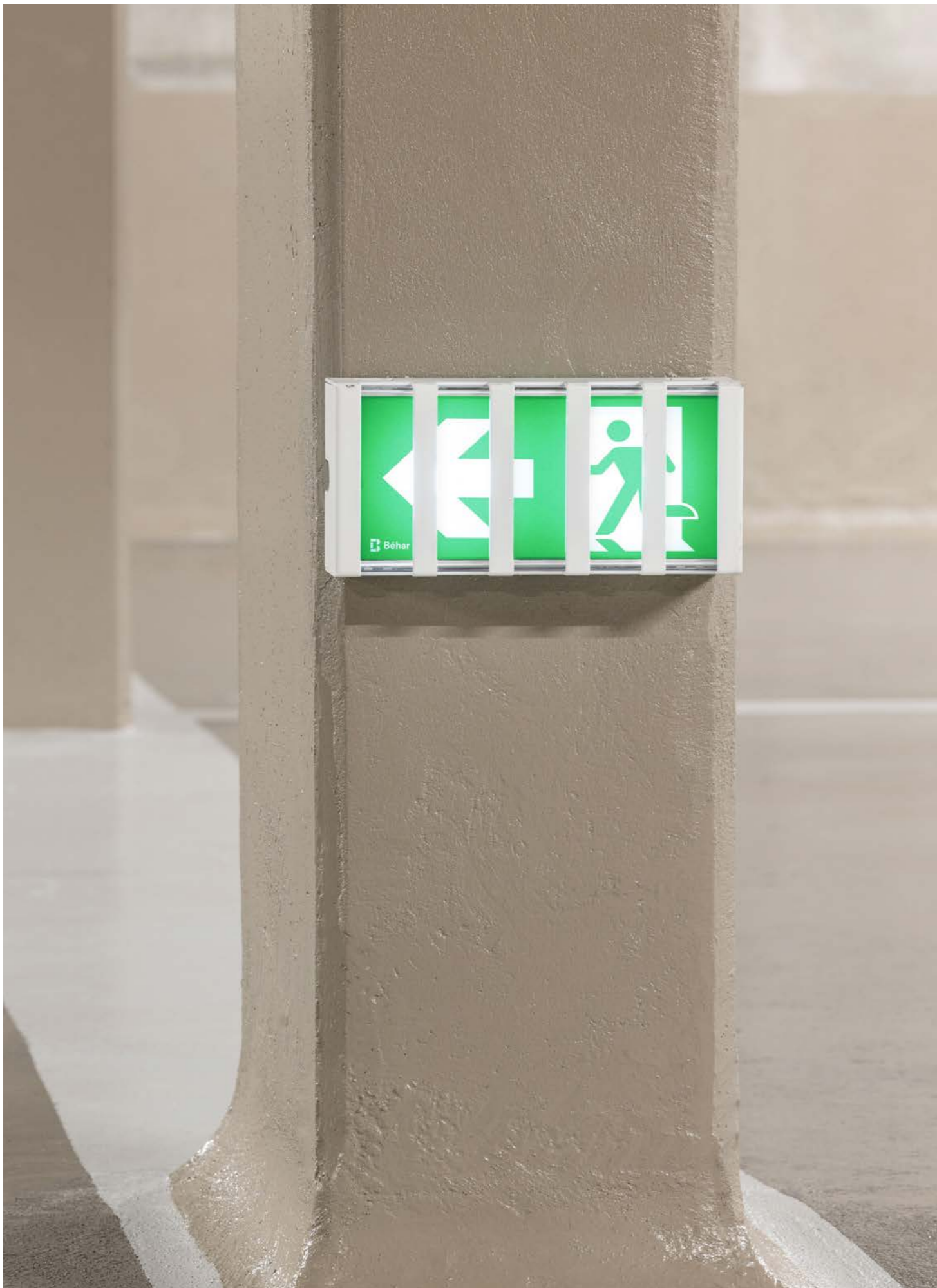
Hôtel Mondrian Bordeaux Les Carmes Parking, Architecture by P. Starck, photo by I. Mathie, Éclat 2 collection
